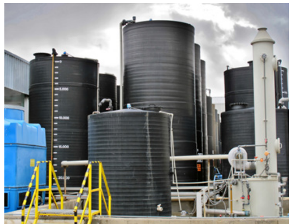
Modern work plant to treat and pack ammonia.
