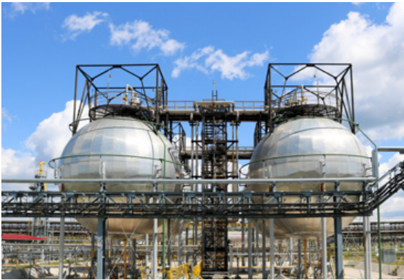
High-pressure iron tank for ammonia storage.
